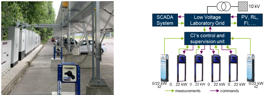
a) Hardware layout in the low voltage Test Grid of the SGL b) Schematic representation of the CI Figure 4: Local CI at Freudenberg Campus of the University of Wuppertal
