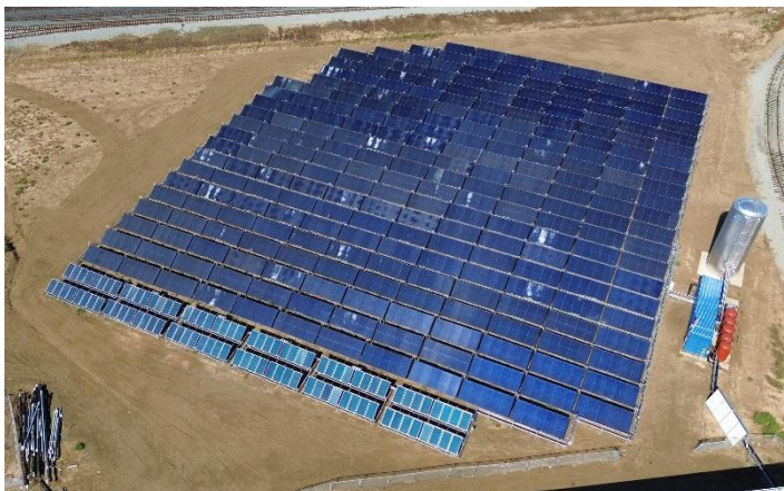
Pic. 1: Overview on Solar System, with collectors, Container and storage tank.
