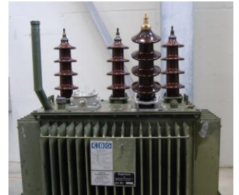
Fig. 1: modified power transformer at IEAN
