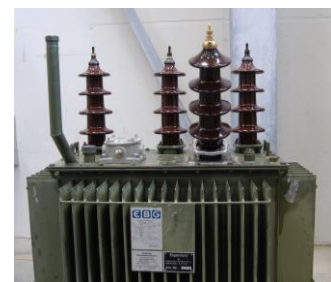
Fig. 1: modified power transformer at IEAN
