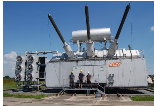
Figure 16: 5-limb 300 MVA power transformer
