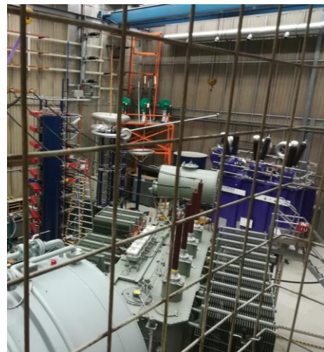
Figure 14: 3-limb 50 MVA power transformer during factory acceptance test
