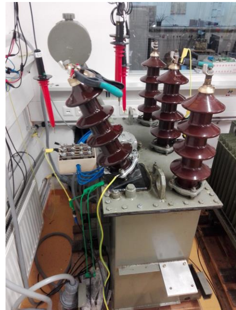
Figure 10: 50 kVA laboratory power transformer
