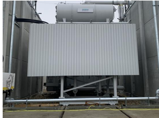
Figure 12: 2-limb 1-phase 183.3 MVA transformer
