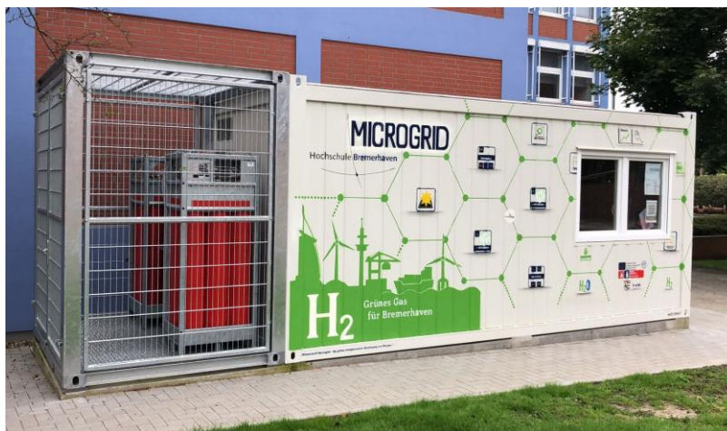
Figure 2: front view of the microgrid container
