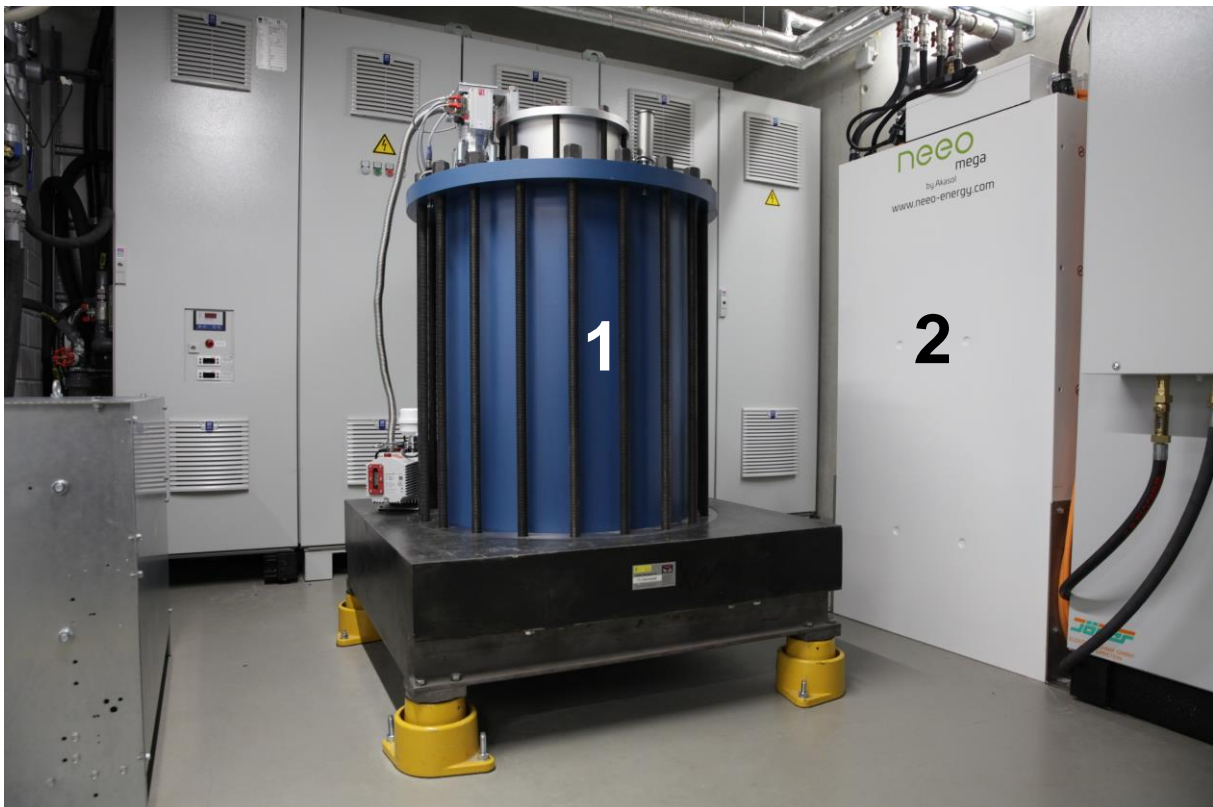
Figure 1 Hybrid Energy Storage System 1: Flywheel, 2: Lithium-ion battery
