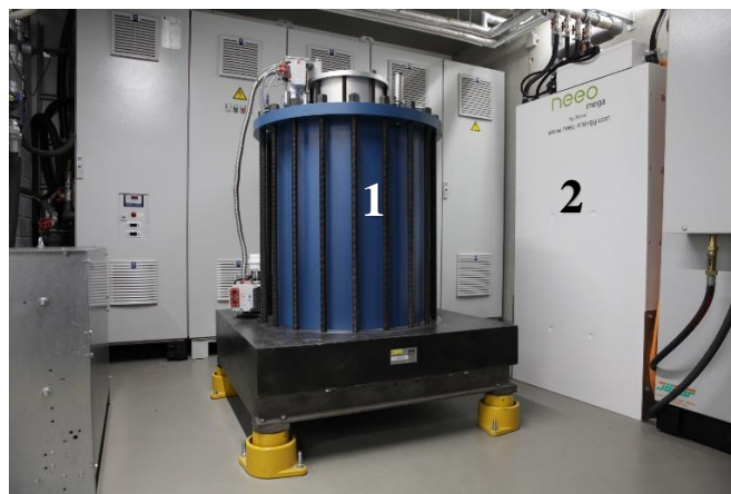
Figure 1: Hybrid Energy Storage System 1: Flywheel, 2: Lithium-ion battery
