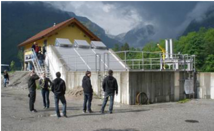
Pumpwerke Hochwasserschutz Golling | Pumping station flood protection Golling
