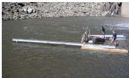
Installation Measstation Grundablass | Installation measurement station bottom outlet
