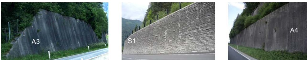
Fig. 4 Gravity walls (left and centre) and one of the anchored walls (right) used in the field study
