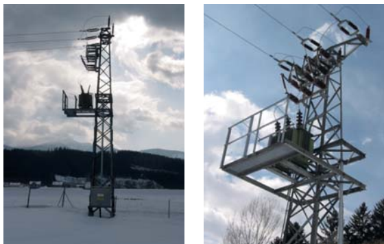
Figure 7: 100 kVA pylon transformer station replaced by a natural ester transformer
