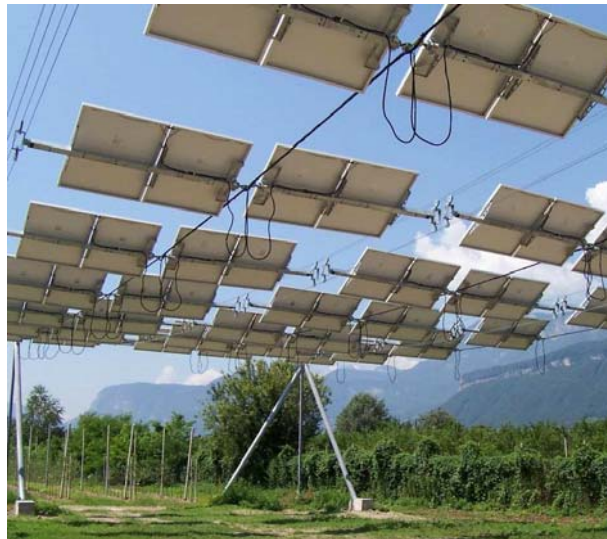
Agro-Photovoltaik Testanlage Laimburg, 2007
