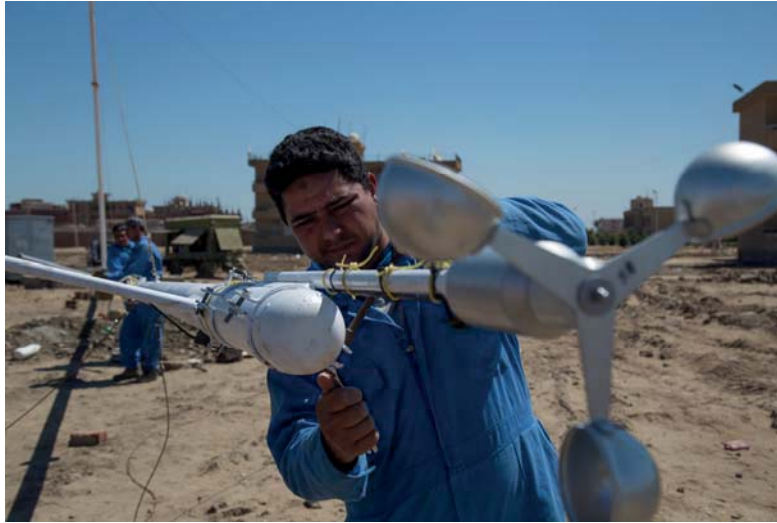
Figure 2: Mounting sensors on locally manufactured 30m measuring pole
