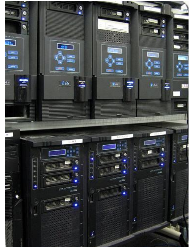
Google Server Farm
